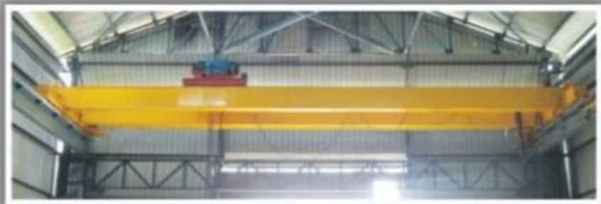
10 TONS EOT CRANE (MODEL: SAI ET 10,000)
