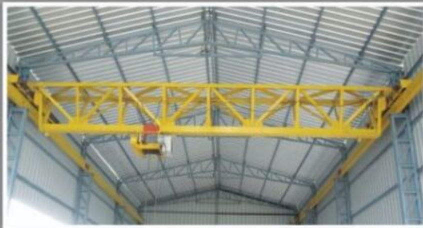
5 TONS EOT CRANE (MODEL: SAI ET 5,000)
